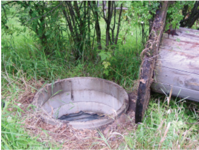
Abandoned wells can act as direct conduits for contaminants from the surface into aquifers.
